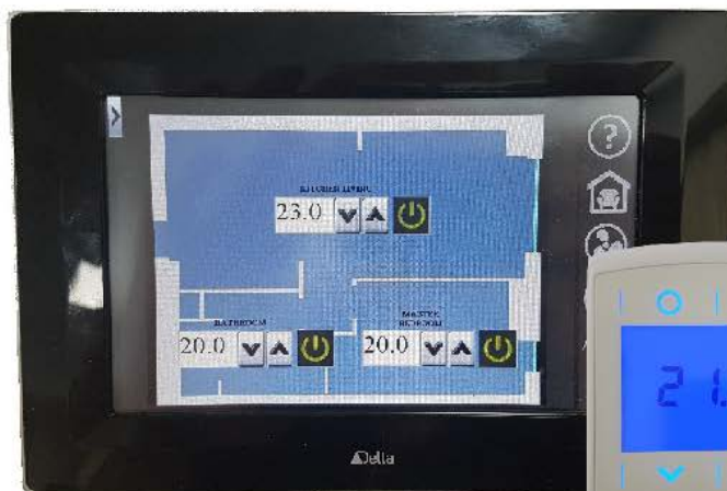
eTCH-7E Control Panel
