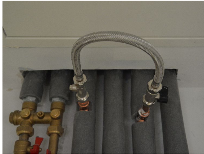
Figure 1.7 - View above HIU unit, with filling loop connected
