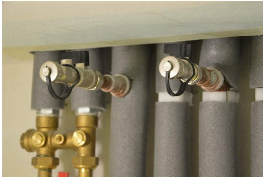
View above HIU unit, the closed valves with caps (A) and (B)
