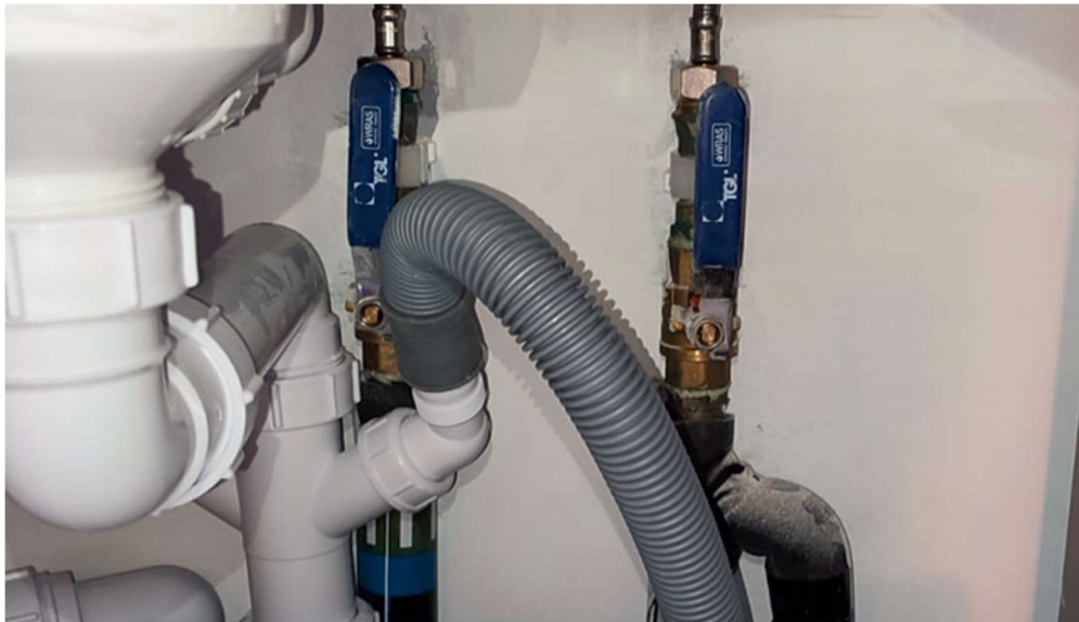
Figure 1.3B - Domestic Water Isolation Valves
