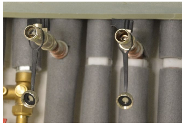
Removed pipe caps are now hanging from the valves
